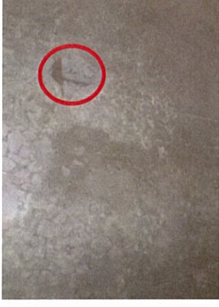
Residence 1950's exposed bars poorly poured concrete surface
