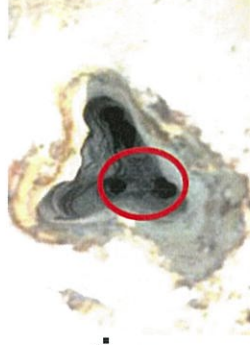
Bars have been tied together and are not welded mesh.
