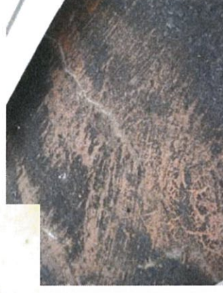
Residence 1950's concrete slab – Does not meet the required Australian Standards
